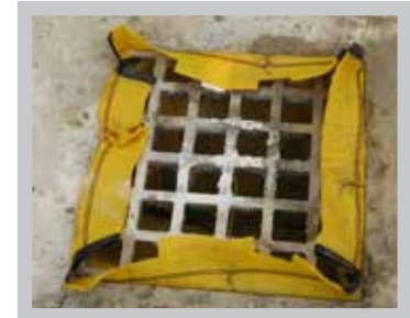
Type A - Installed.
