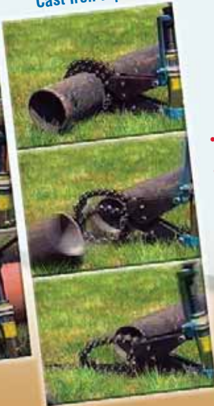
Cast Iron Pipe
