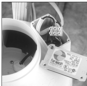
Romex wiring – Top View
