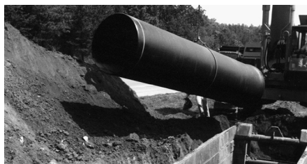
This 30" AMERICAN Ductile Iron Fastite joint treated-water transmission main was furnished and installed—as is most ductile iron pipe—with standard asphaltic coating approximately one mil thick on the outside.
