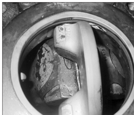
Figure 1 - shows the valve properly clamped in place
